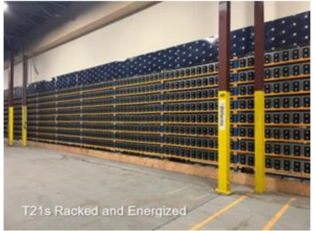
T21s Racked and Energized
